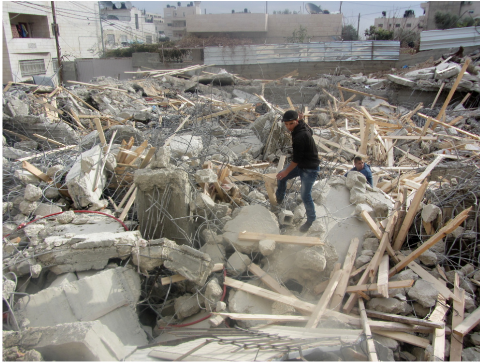
Home demolition in East Jerusalem (photo, 'Amer 'Aruri, B'Tselem researcher, http://www.btselem.org/photoblog/20140209_jerusalem_demolitions , via Wikimedia Commons)
