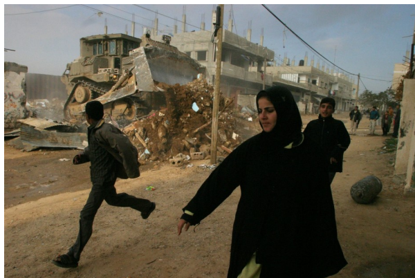
House demolition in Rafah Seam Zone by an armored Caterpillar D9. (Photo: Khalil Hamra)
